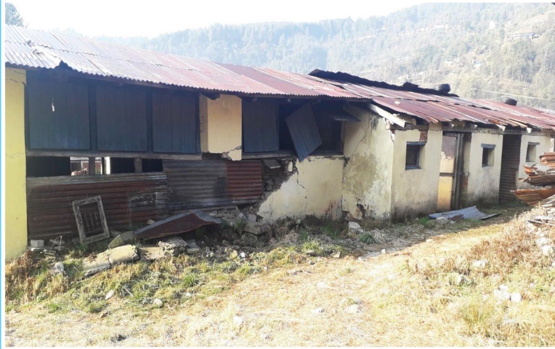
Cows also are waiting for refurbished shed
